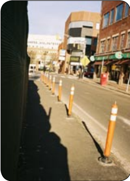
Bollards or delineator posts are currently used in Cambridge, MA to define a sidewalk during construction.
